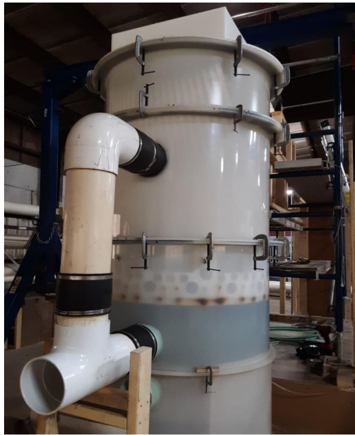
Figure 6 Outlet and Bypass Piping
